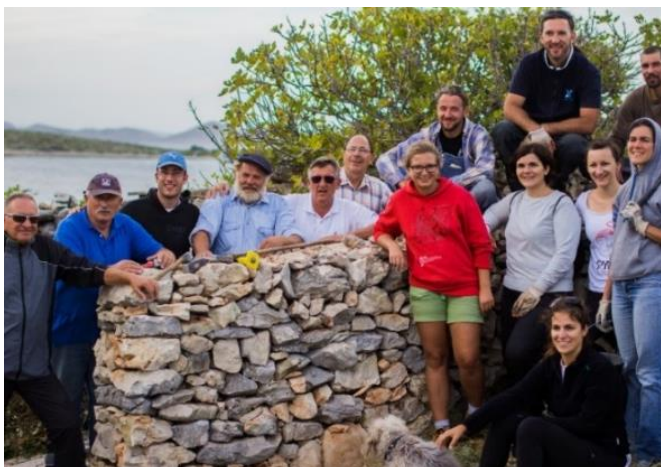
Figure 2 As a bond of social capital and sustainability, dry stone walls, and their restoration are a central part of the Oživi održi otok Action plan for sustainable use of resources of Murter region.
